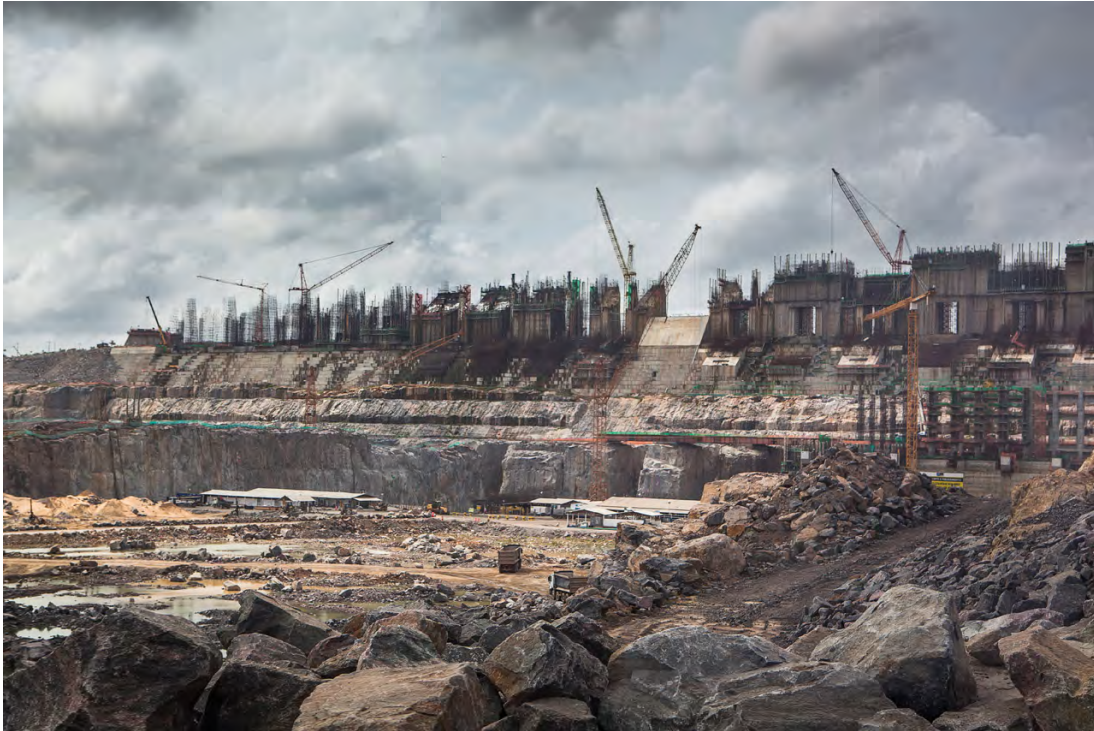
Construction of Belo Monte Dam, on the Xingu river, Belo Monte Site. Altamira, Pará, Brazil. Credit line: © Carol Quintanilha / Greenpeace
