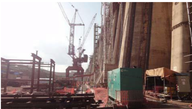
Photo 48: Right Bank Power House with many safety hazards.
