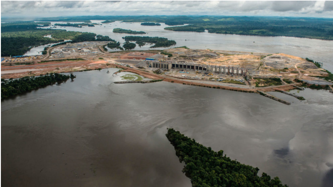
The Belo Monte Dam under construction on the Xingu River, a tributary of the Amazon, in 2015. FÁBIO NASCIMENTO/GREENPEACE
